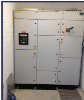
SUBSTATION & SWITCH ROOM
