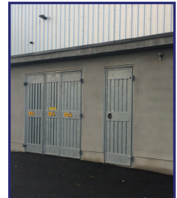
SUBSTATION & SWITCH ROOM
